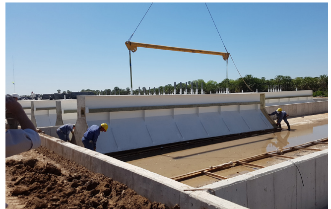
Reactors (Gran Resistencia plant)
